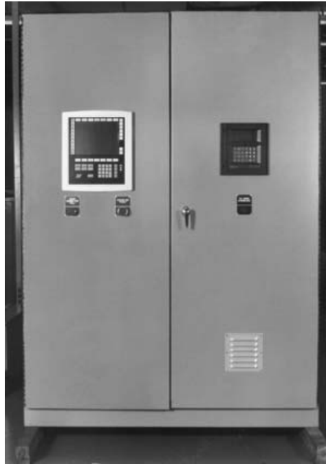
FIGURE 21.6 Pipeline compressor panel (programmable logic controller and temperature scanner) front panel view. (Courtesy of Advanced Control Engineering Services).
