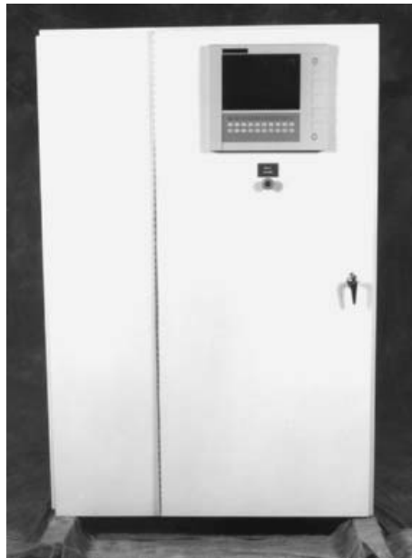
FIGURE 21.3 Pipeline compressor panel (programmable logic controller panel) front view.
