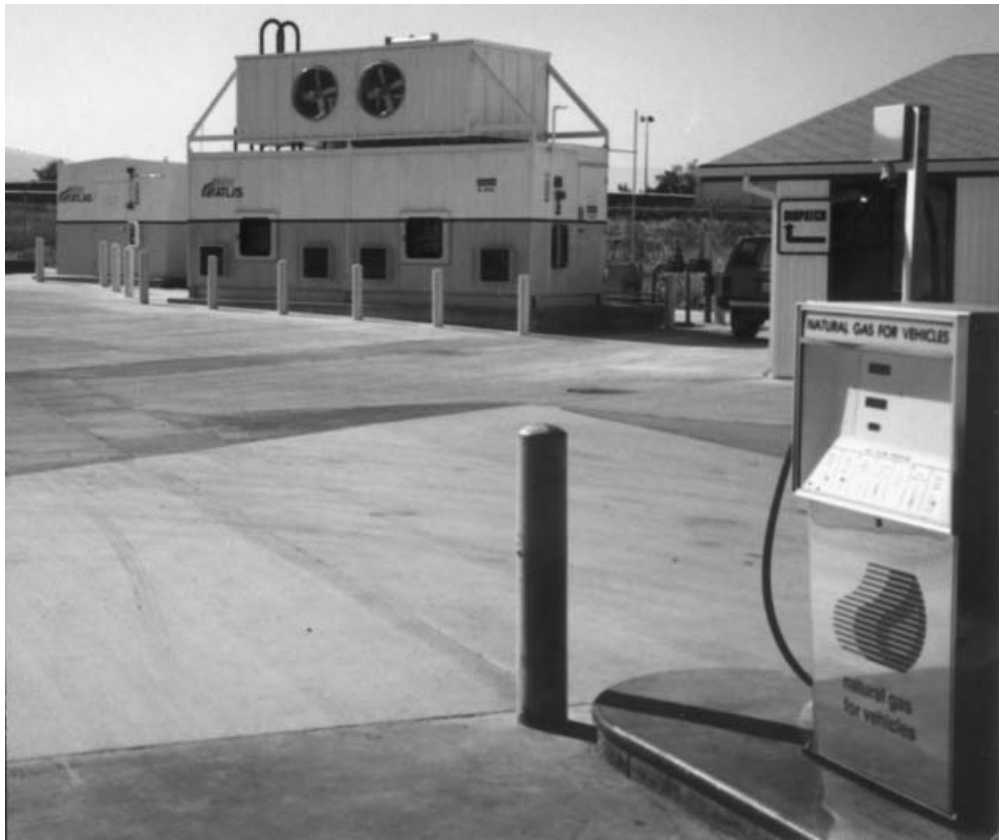
FIGURE 8.1 Compressed natural gas refueling station ( courtesy of IMW Altas Inc. ).
